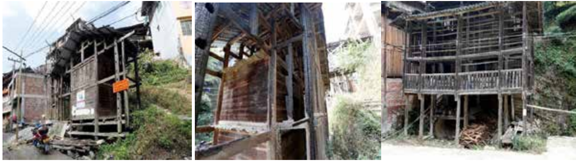
Fig. 1. Dilapidated Dong wooden buildings.
