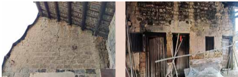
Fig. 3. Missing roof and walls of He ancestral hall.
